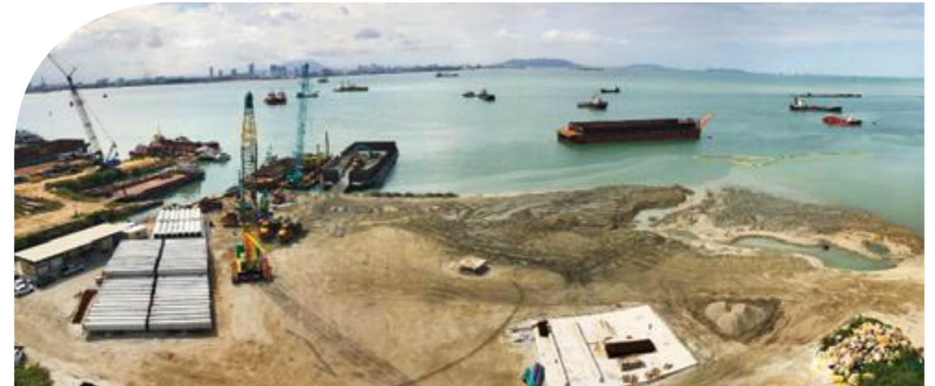
Penang Submarine Pipeline
