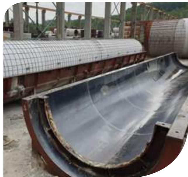
Penang Submarine Pipeline
