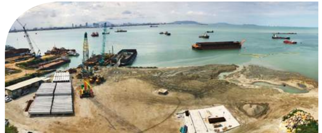
Penang Submarine Pipeline
